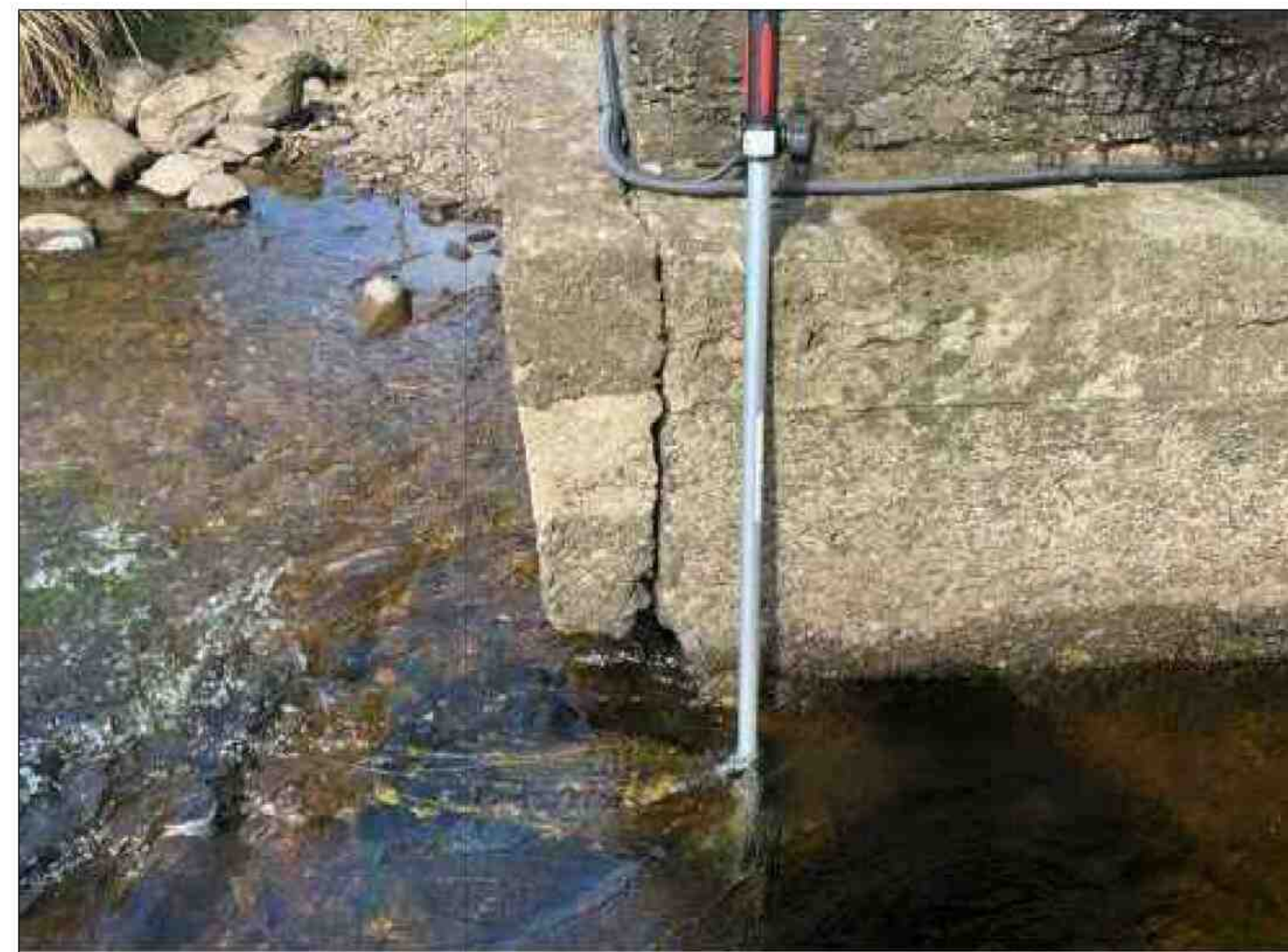
8. CRACKING AND UNDERMINING TO THE WEST END OF THE NORTHERN PIER SCOUR PROTECTION
