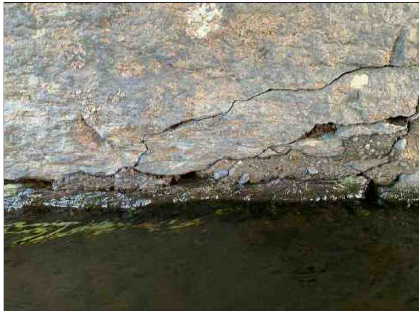
7. SETTLEMENT CRACKS TO SOUTHERN PIER MASONRY
