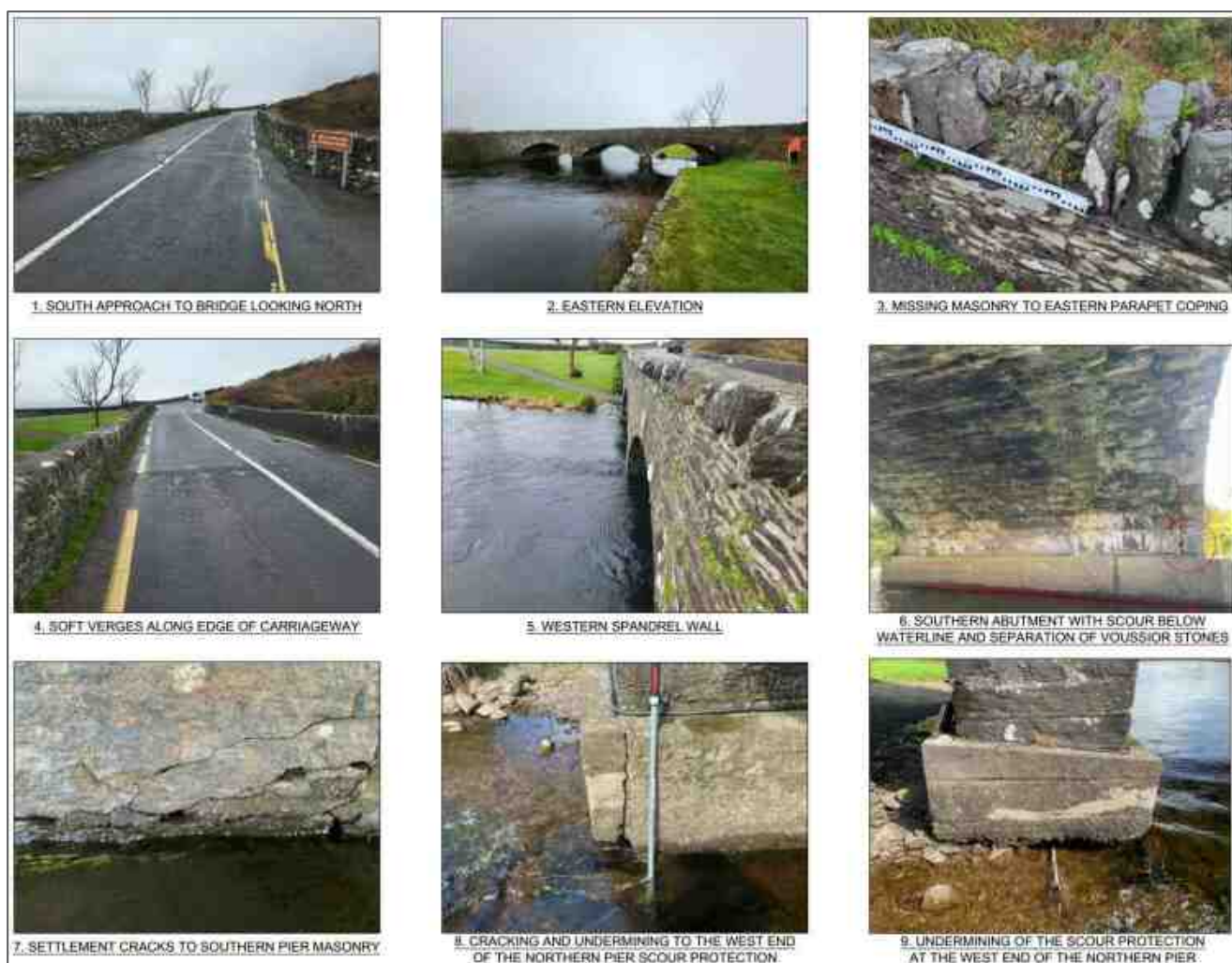
Figure 1-2 - Damage noted during inspection (see at original scale in Appendix A).
