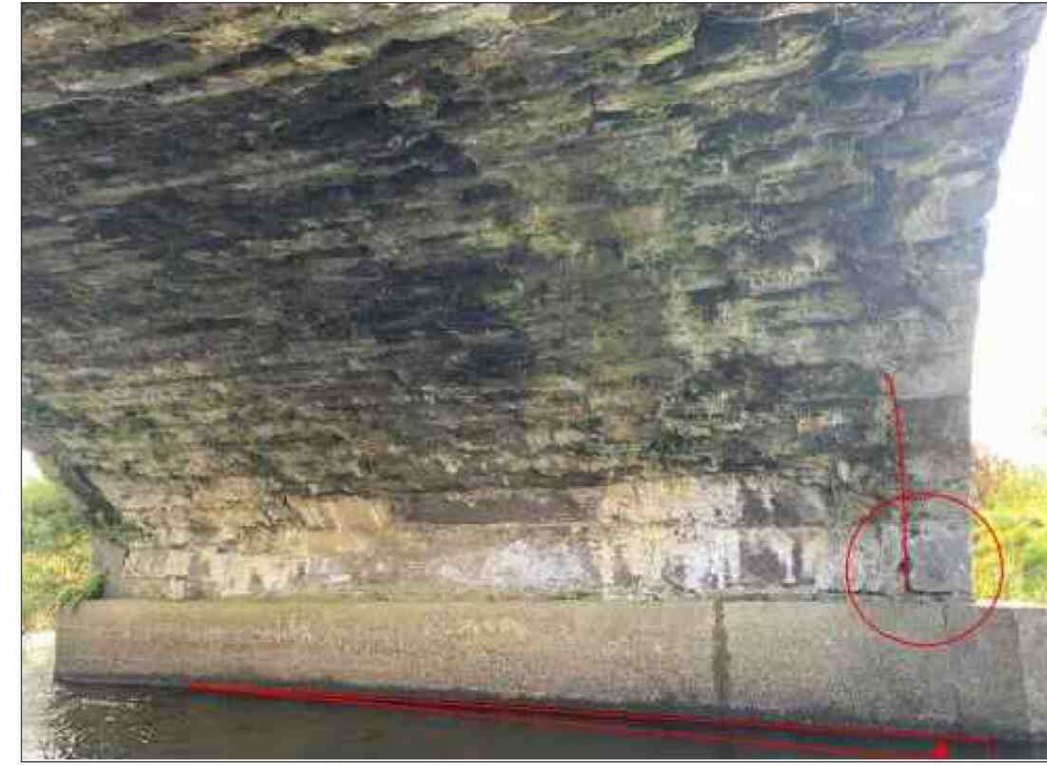
6. SOUTHERN ABUTMENT WITH SCOUR BELOW WATERLINE AND SEPARATION OF VOUSSIOR STONES
