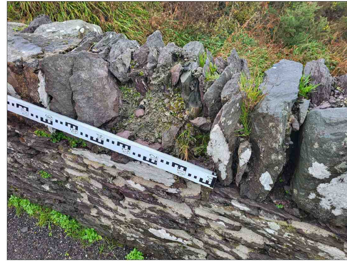
3. MISSING MASONRY TO EASTERN PARAPET COPING
