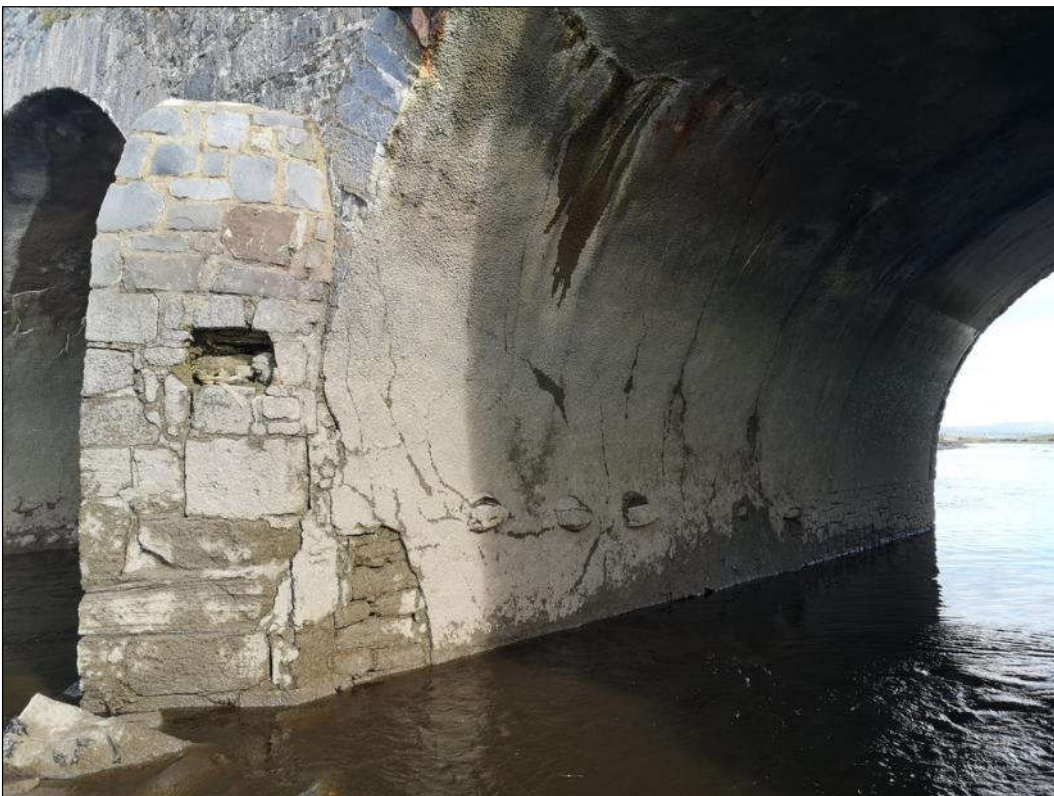
Plate 1.14 Masonry loss and separation to the west cutwater of pier 2.
