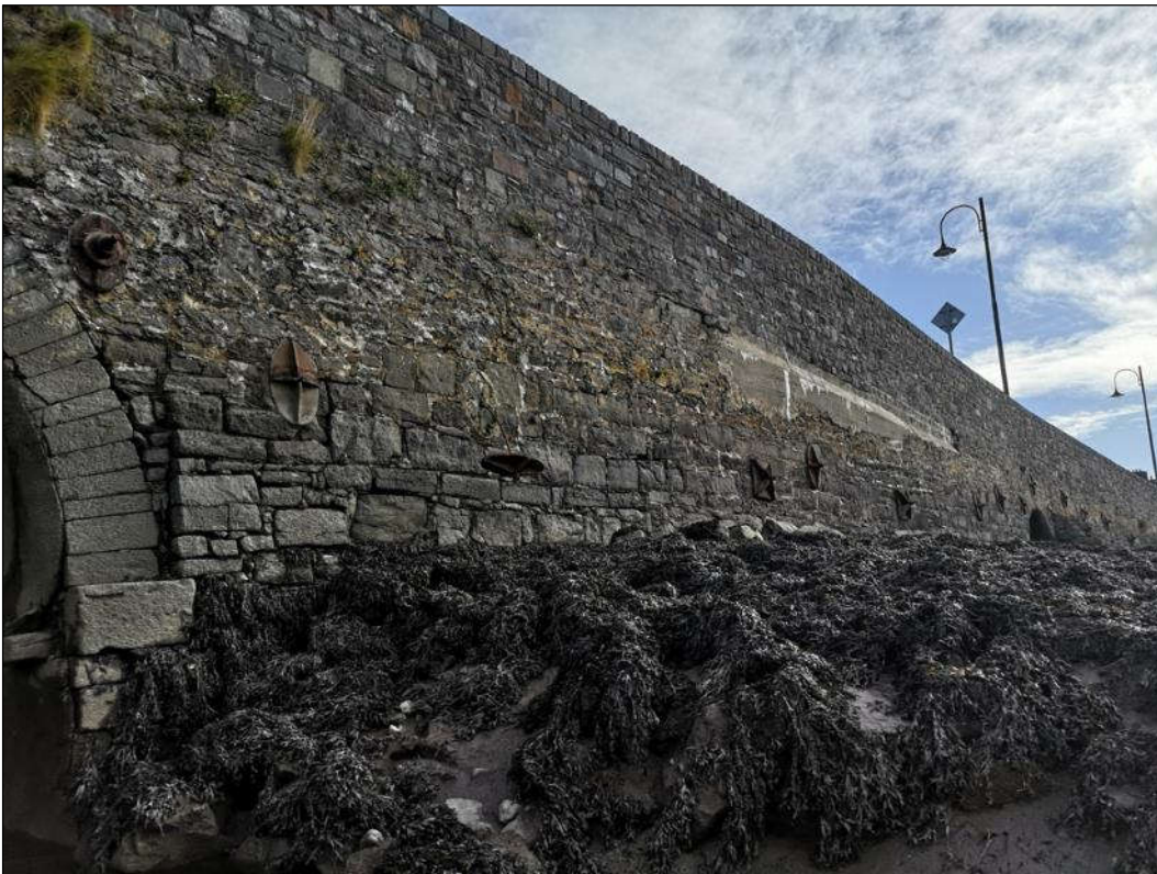
Plate 1.6 View of the SW wing wall with detached parrass plate and previous concrete repair evident.
