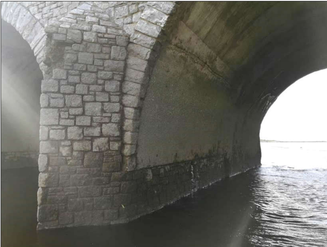
Plate 1.13 Missing masonry to the east cutwater of pier 2.
