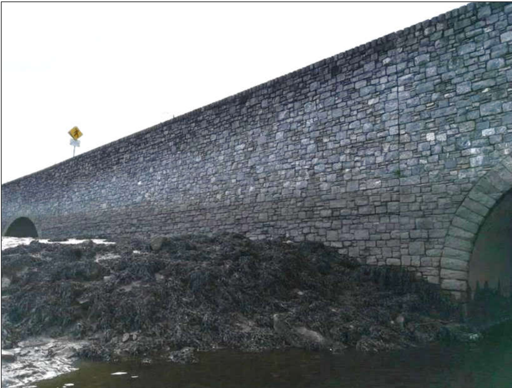
Plate 1.7 View of the SE wing wall with high tide staining evident.
