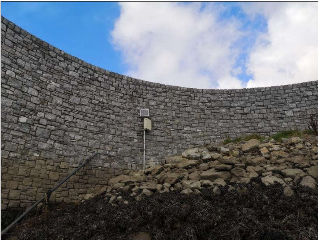
Plate 1.8 View of the NE wing wall with high tide staining evident.
