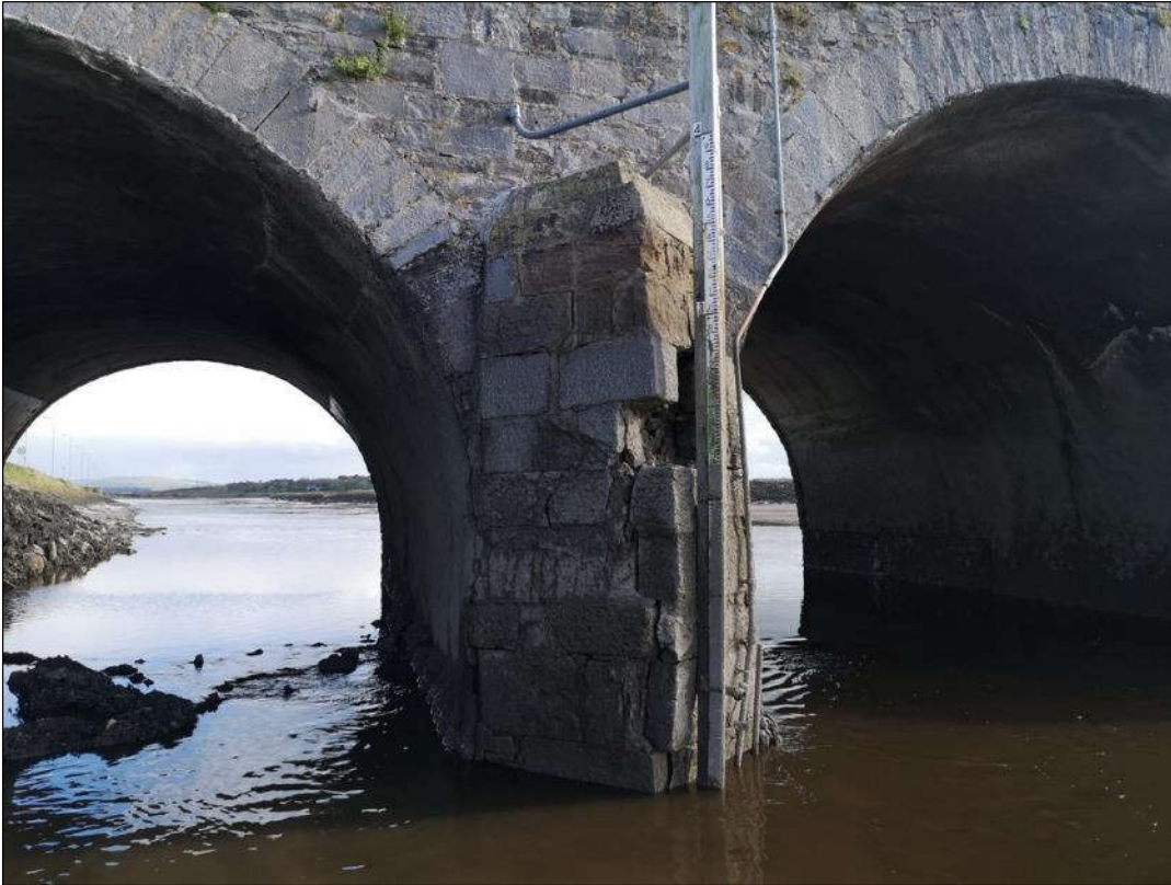
Plate 1.11 View of the west cutwater of pier 1 with cracked and missing masonry evident.
