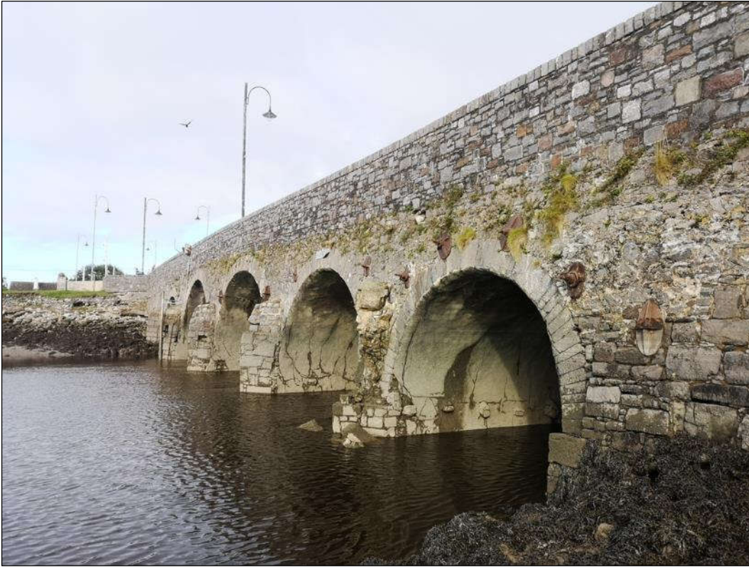
Plate 1.9 View of the west spandrel wall with vegetation growth evident.
