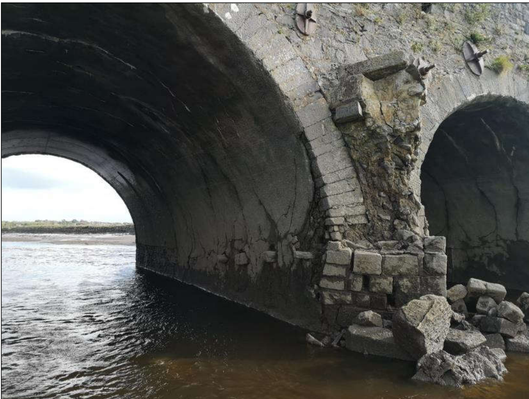
Plate 1.16 Collapsed west cutwater of pier 4.
