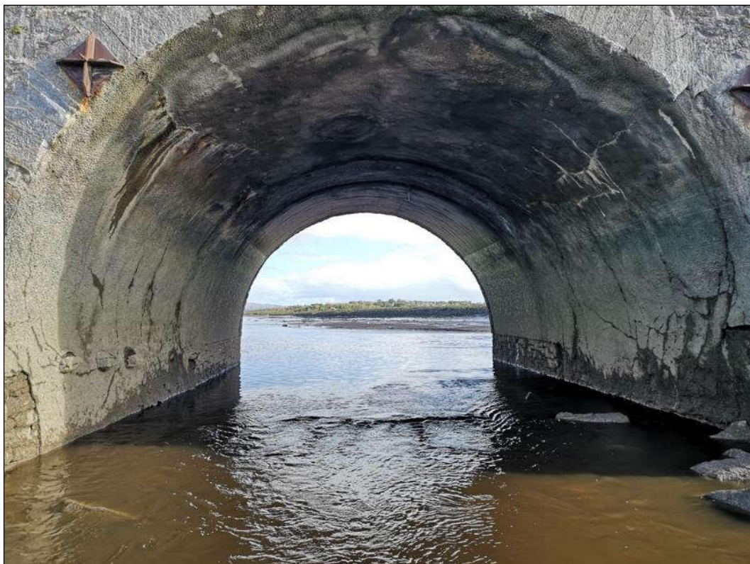
Plate 1.18 View of arch barrel in span 3 with extensive cracking to the gunnite layer at both quarter points.
