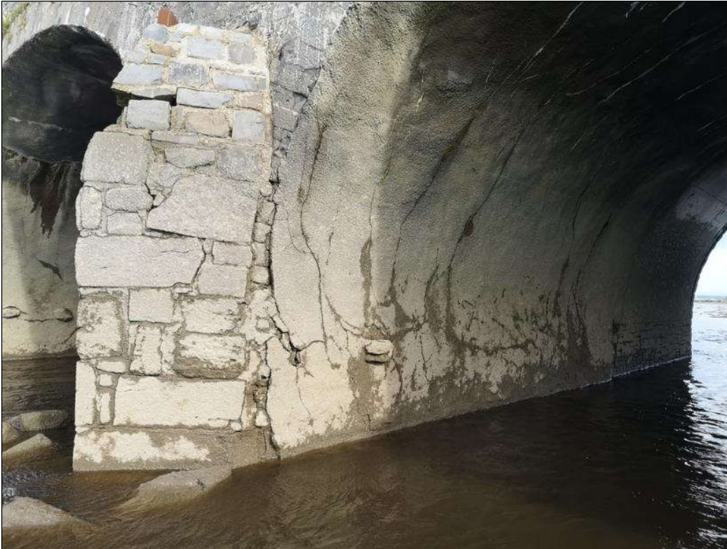
Plate 1.15 View of the west cutwater of pier 3 with masonry loss evident and cracking to the gunnite layer on the south face.
