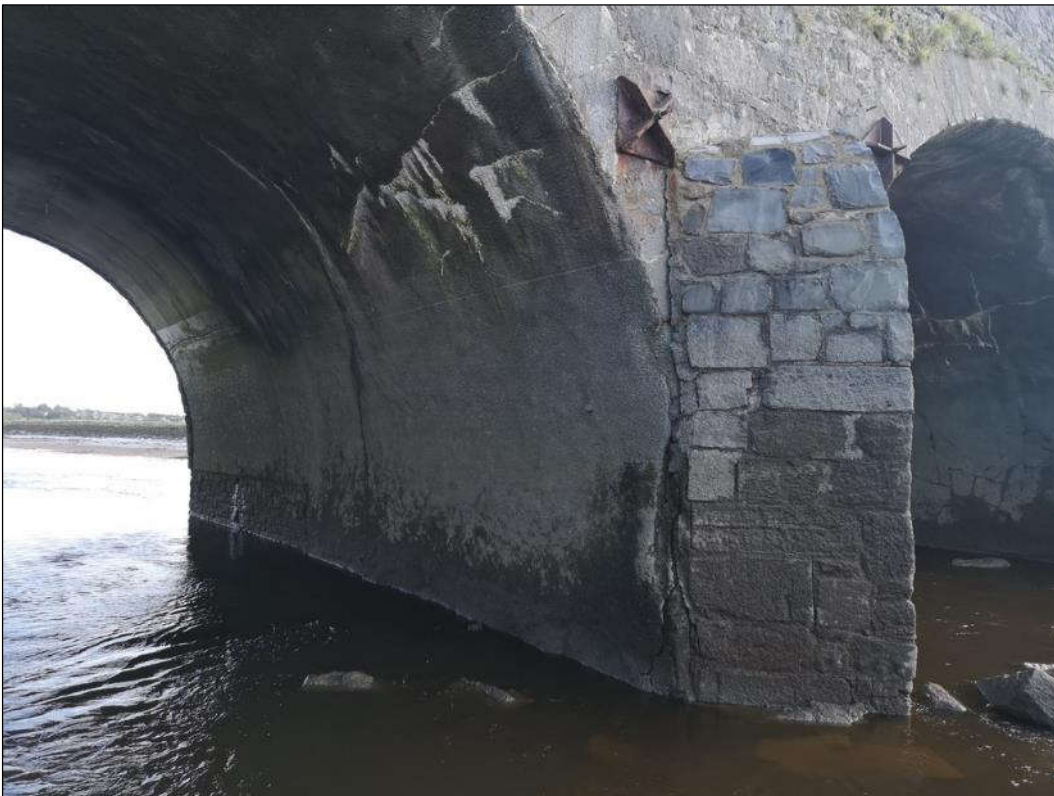
Plate 1.12 View of the north face of pier 2 with 10mm wide vertical crack evident from quarter point of arch down to riverbed at middle of structure.
