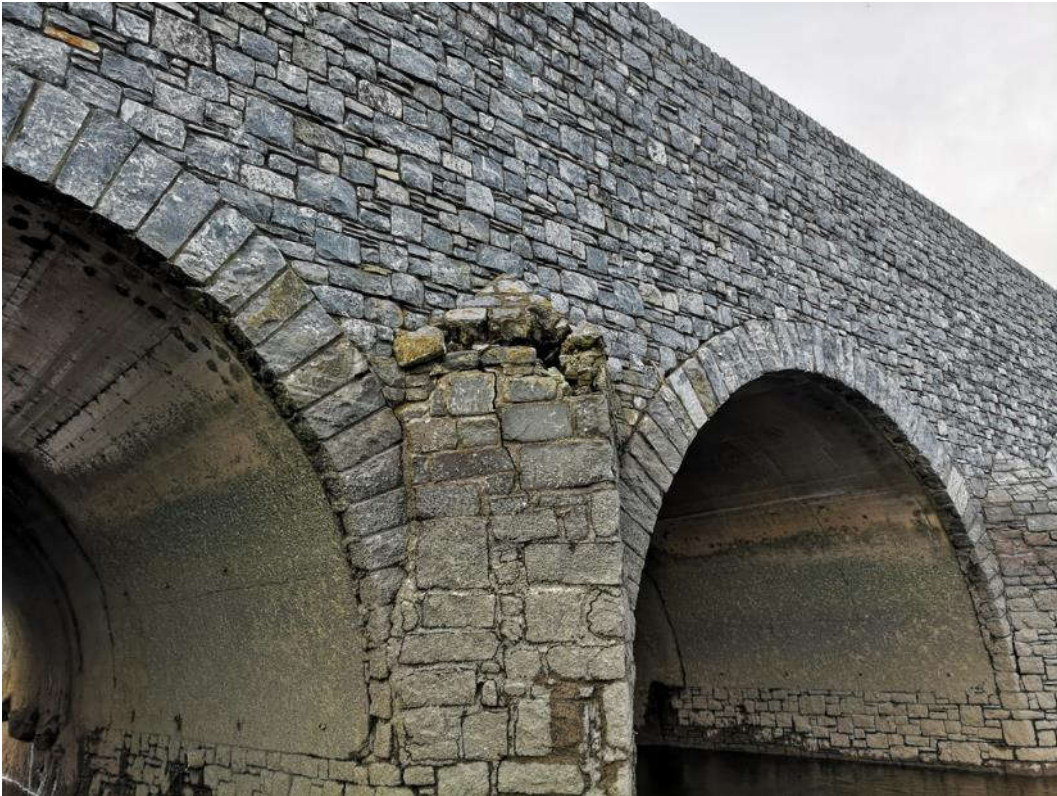
Plate 1.17 Missing and cracked masonry to the east cutwater of pier 4.
