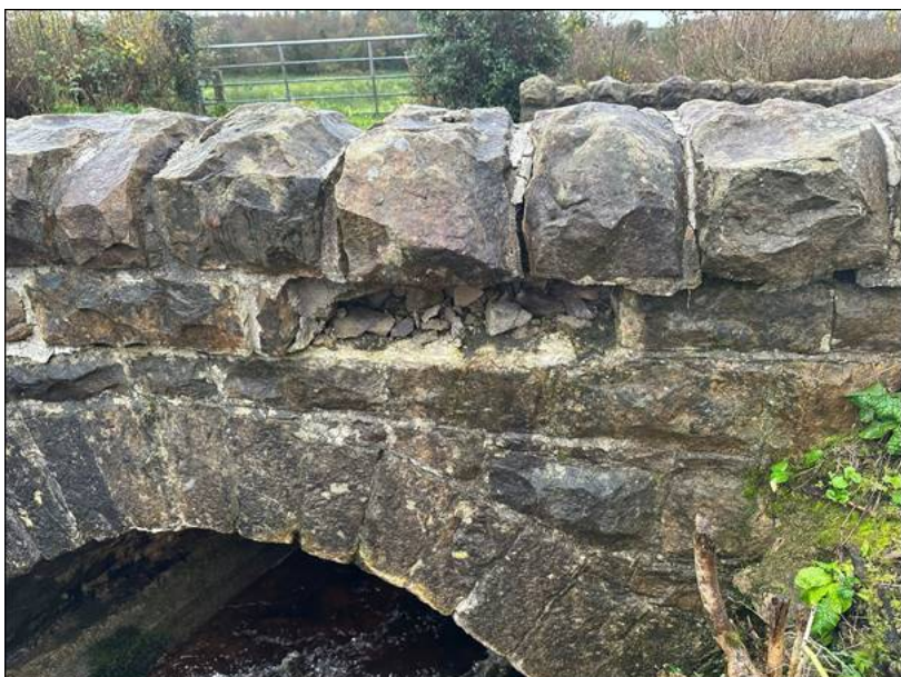
Figure 4: Missing fascia on riverside face of the damaged parapet.
