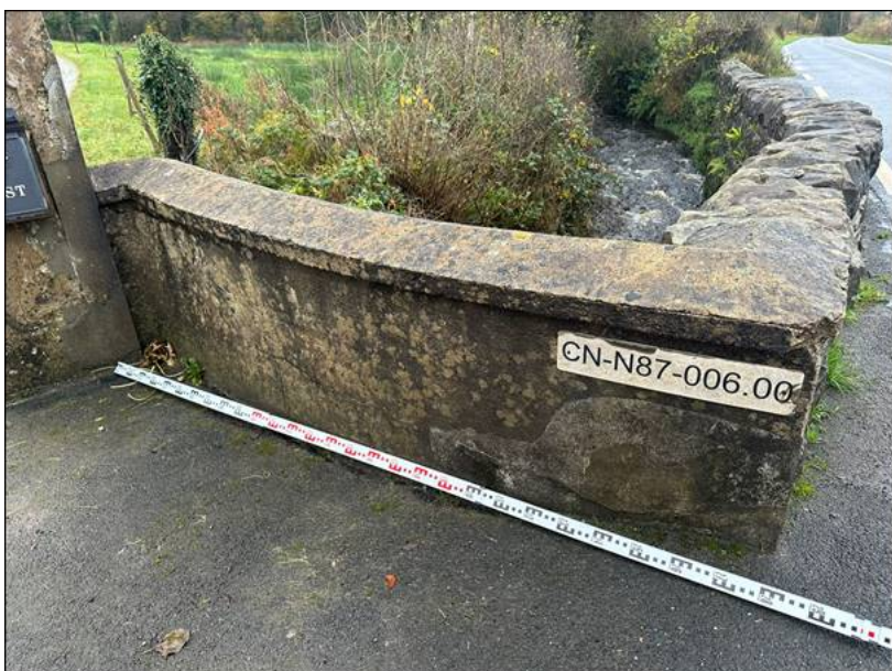
Figure 5: Damaged entrance wall adjoining the north-eastern parapet of Tawnagh Bridge.
