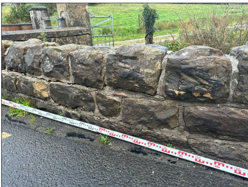
Figure 3: Damaged parapet to be rebuilt.
