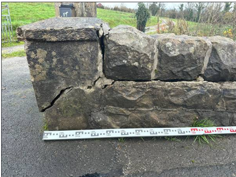
Figure 2: Damaged coping (right) attached to the damaged entrance wall (left) adjoining Tawnagh Bridge.
