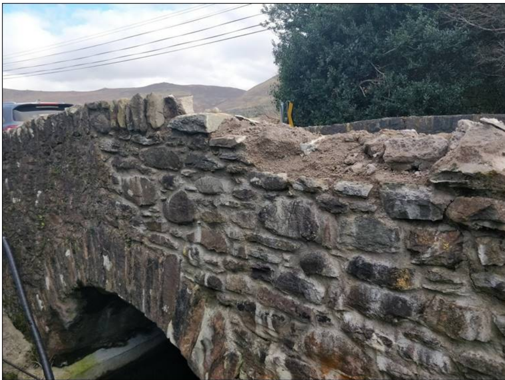
Figure 3: The damaged parapet wall on the water-side of the bridge.
