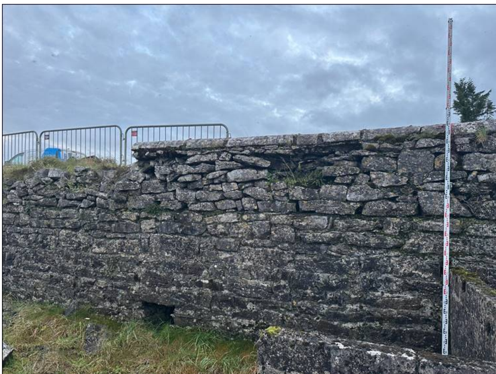
Figure 3: Second damaged section of the parapet to be repaired.
