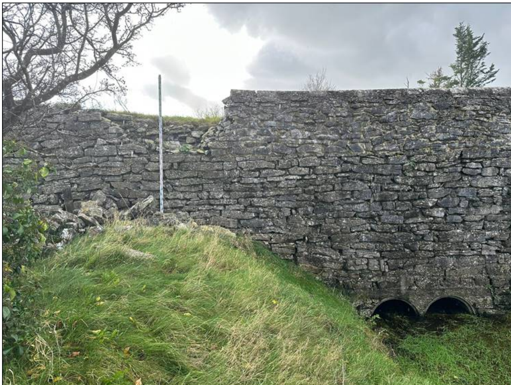
Figure 2: First damaged section of parapet to be repaired.
