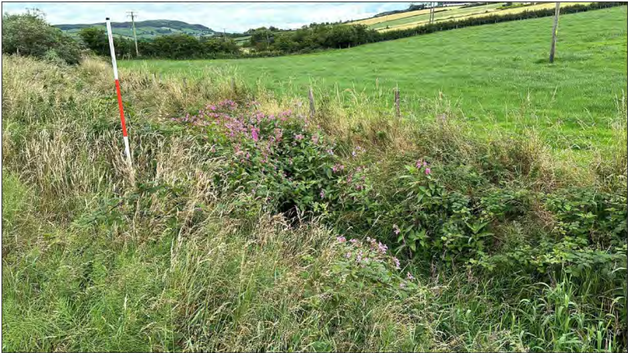
Plate 4.11 - Himalayan Balsam at Cavan Bridge Culvert.
