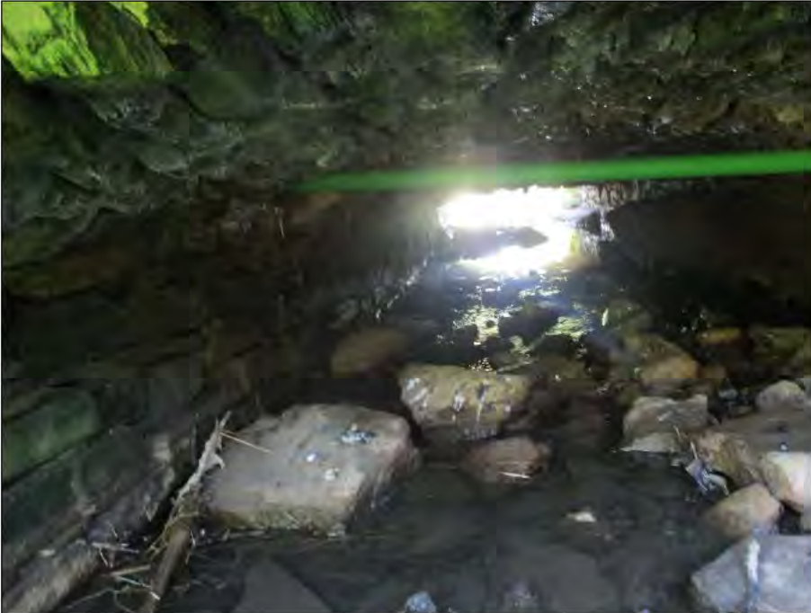
Plate 4.1 - The stream channel flowing beneath Cavan Bridge Culvert, large boulders present. There is also a fibre optic cable running under the bridge.
