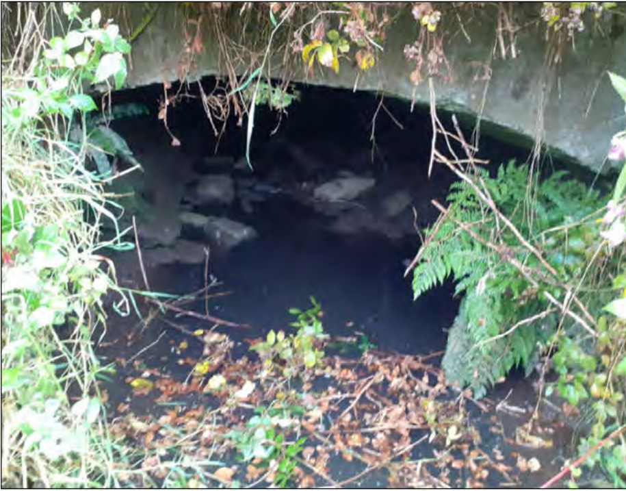
Plate 4.8 - Downstream face of bridge with shallow concrete arch extension to original masonry structure.
