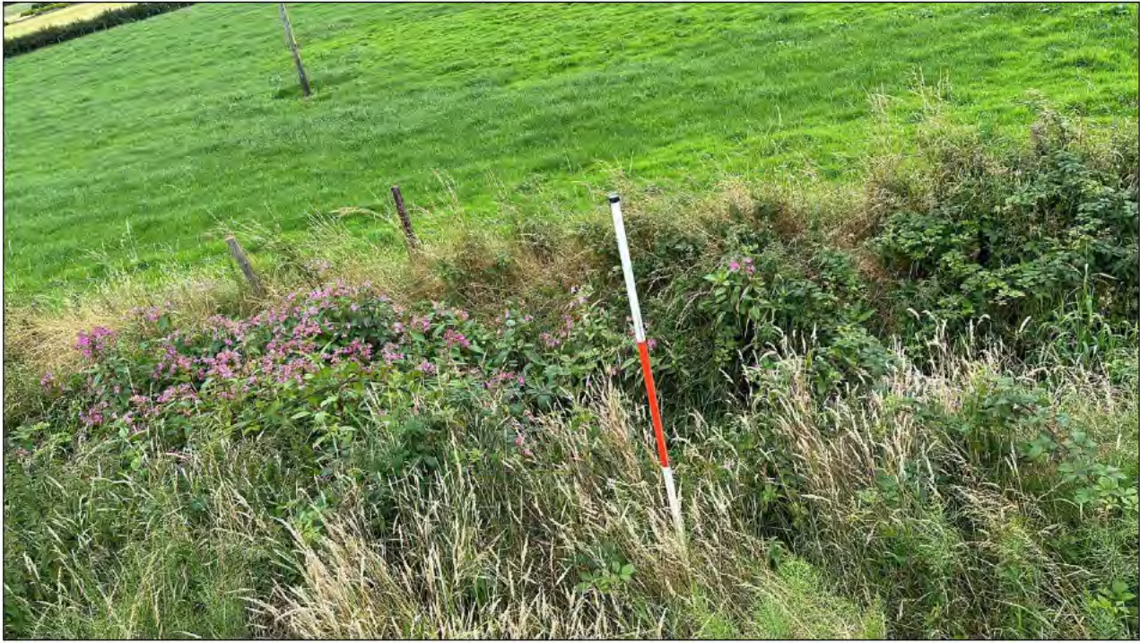
Plate 4.10 - Himalayan Balsam at Cavan Bridge Culvert.
