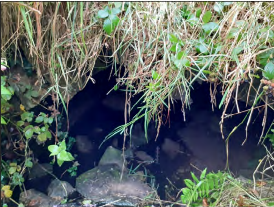
Plate 4.7 - Upstream face of masonry section heavily overgrown with vegetation. Some arch facing stones have collapsed.
