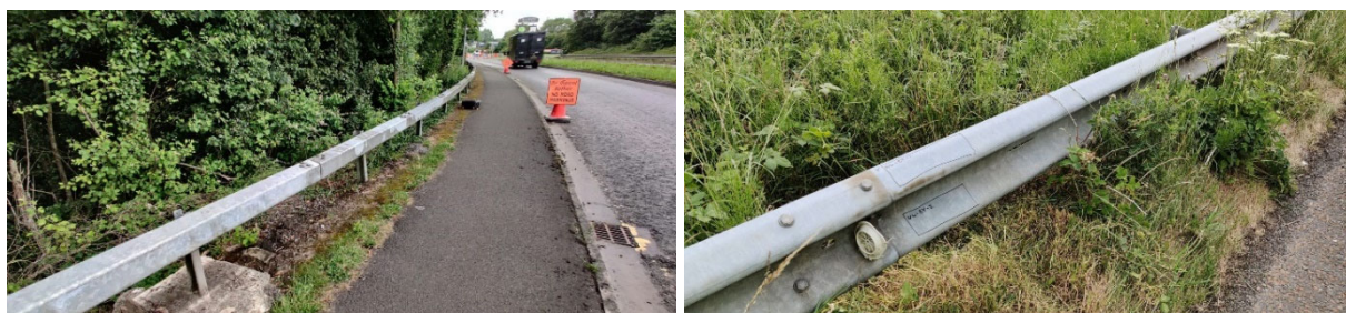
Figure 2.1 – Examples of old Open Box Beam (OBB) and Tensioned Corrugated Beam (TCB) barriers
