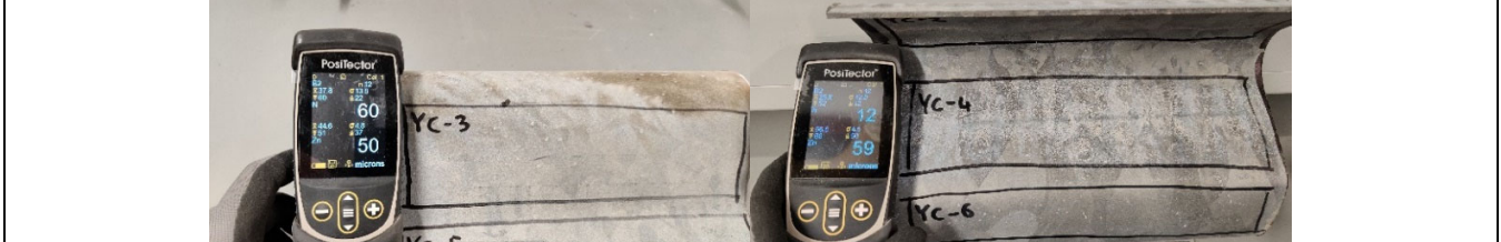
Figure 2: Example of measurement on area '3' (left) and '4' (right) for crash barrier labelled 'N59-GY-SB09A'.
