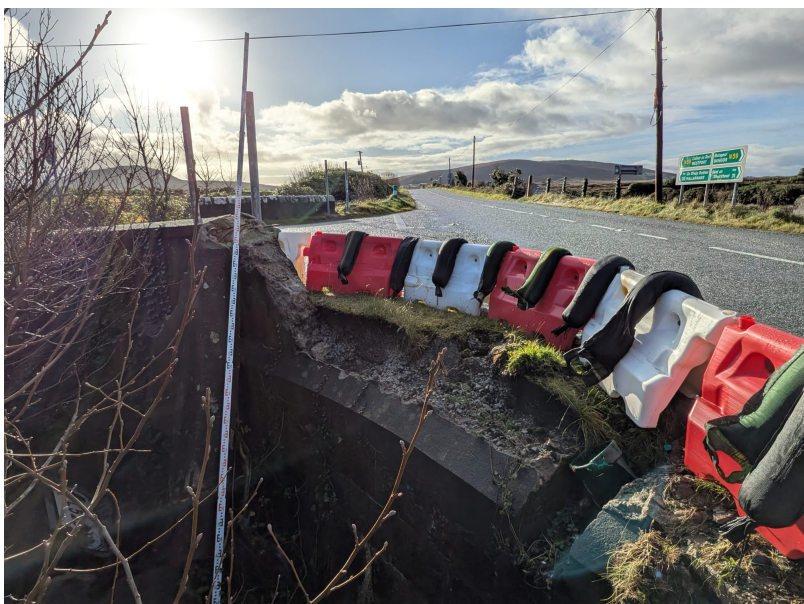
Figure 3: Damaged section of the parapet with missing blockwork as viewed from the riverbank.
