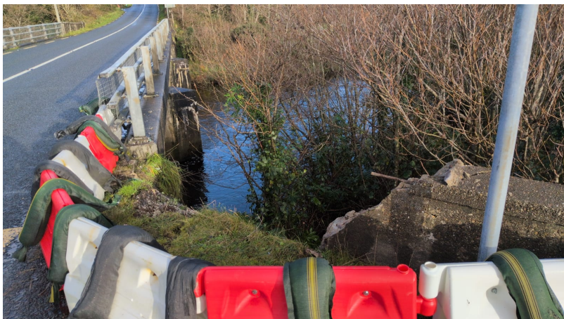
Figure 2: Damaged section of parapet with missing blockwork and damaged steel barrier as viewed from the roadside.
