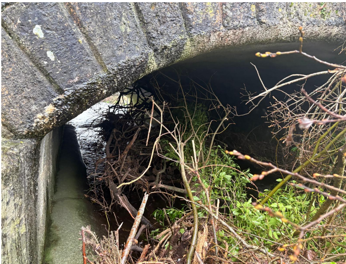
Figure 3: Debris trapped underneath one of the arches of the bridge.
