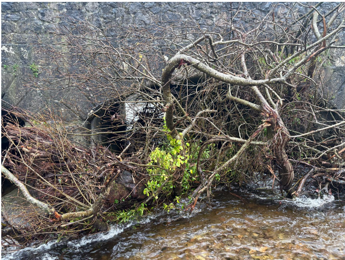
Figure 2: Debris trapped on upstream side of the bridge.
