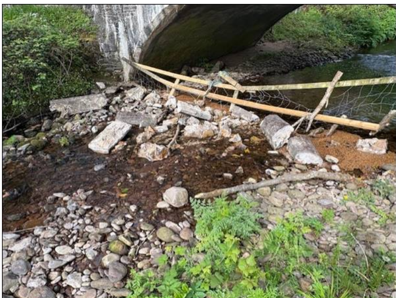
Figure 3: Debris within the River Owenashad.
