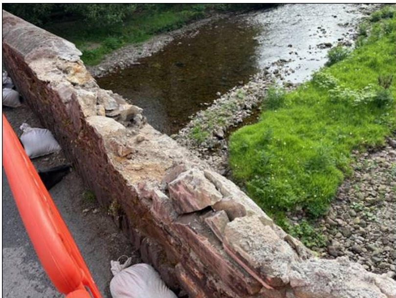
Plate 2 – View of the damaged area, dry works area and the Owennashad River.
