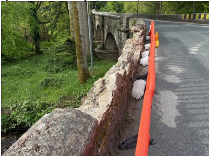
Figure 2: Damaged section of parapet.
