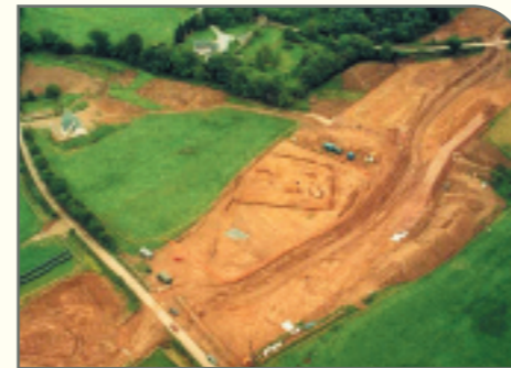
Aerial view of early medieval enclosure uncovered at Ballynacarriga . (Photo A.C.S. Ltd.)
