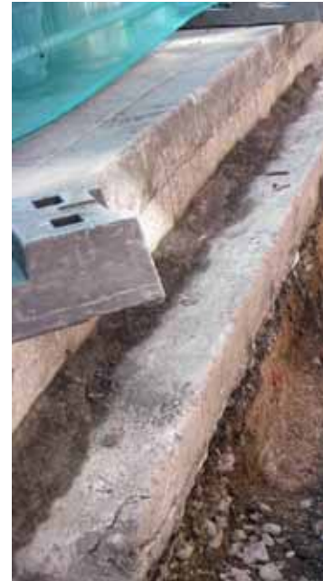
Plate 3: View from east of excavated pipe trench. Note demolition material C.5 in south of trench
