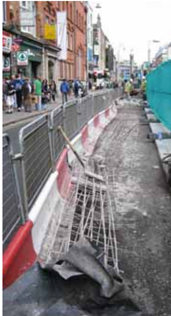
Plate 1: View of Abbey Street Stop works area from west, post-removal of temporary surface
